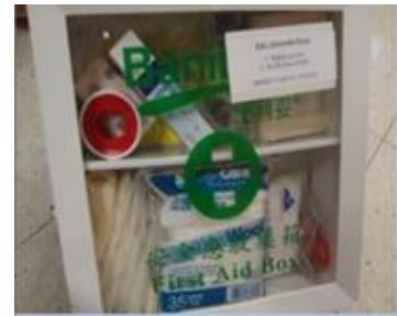
First aid boxes are provided in the units and Facilities Management Office
